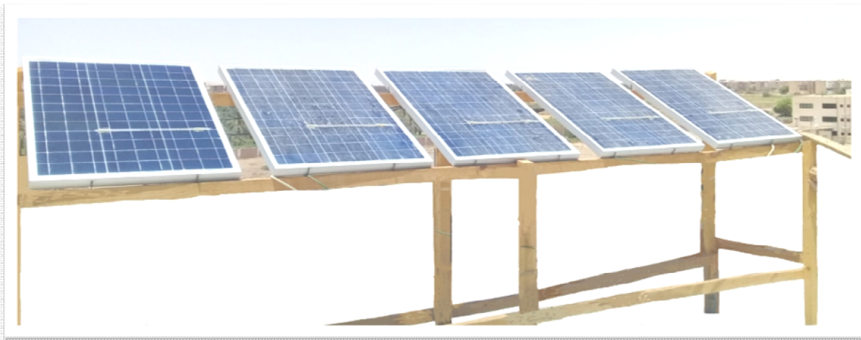
Figure 3. Five photovoltaic (PV) panels fixed at 30 degrees facing the sun southward at El-Kharga Oasis.
